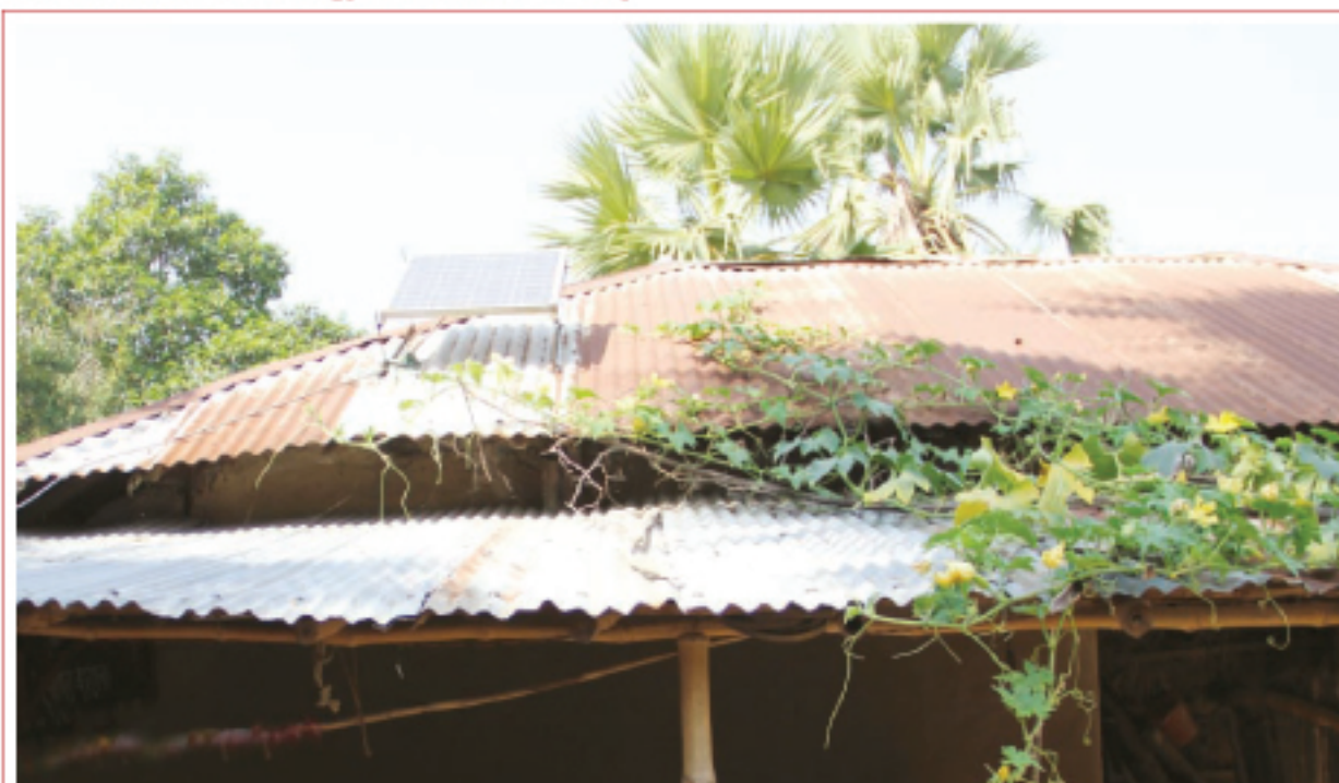
Solar PV panel installed at model climate resilient community in Godagari : photo ©Sajjadul/LoCAL-UNCDF
