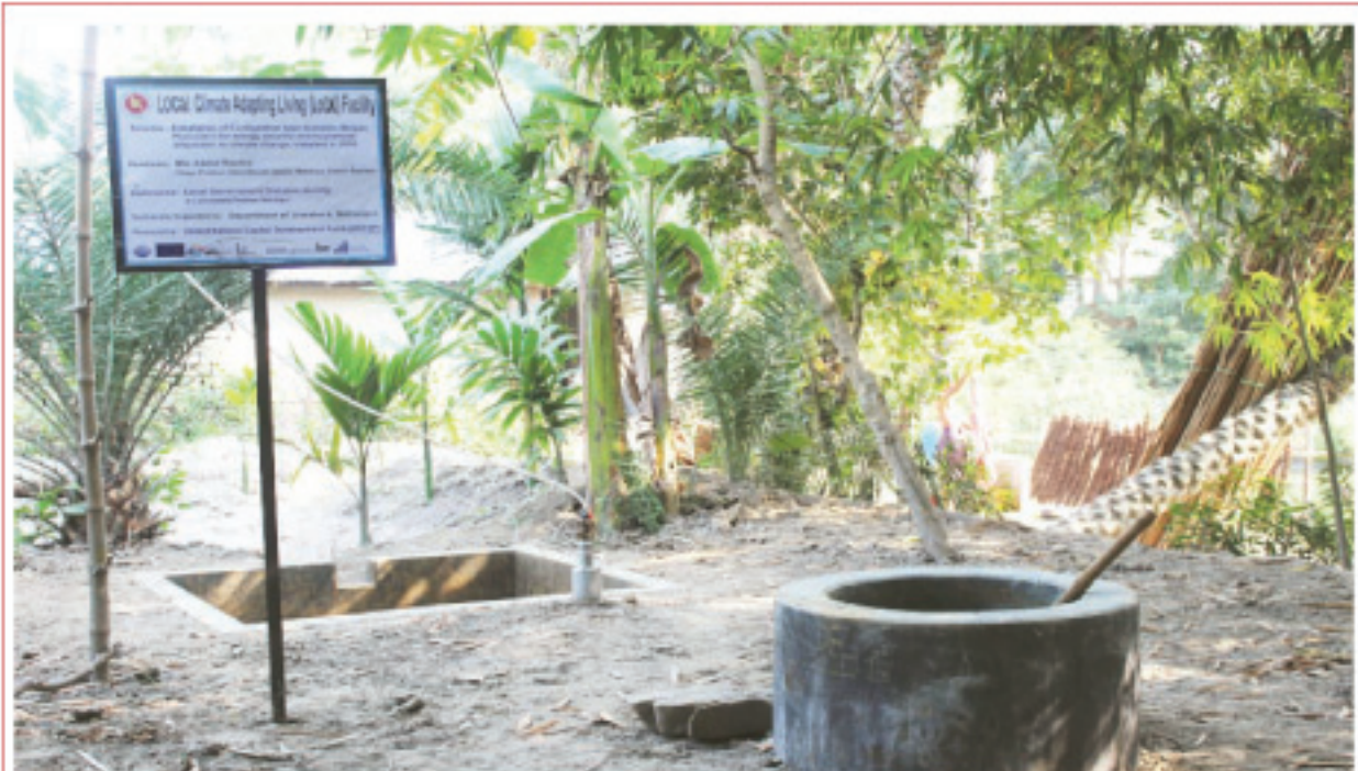
Biogas digester installed with model climate resilient community : photo ©Sajjadul/LoCAL-UNCDF
