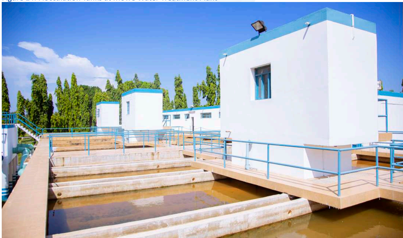
Figure 14: Flocculation Tanks at Mowe Water Treatment Plant
